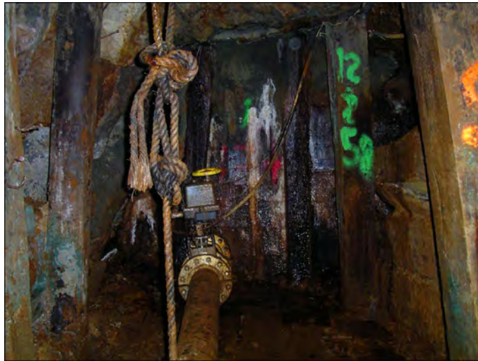
BULKHEAD AND VALVE (2008)
